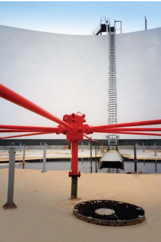
Typical foam manifold
